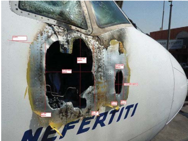
Figure 2. Fire burned through the skin of EgyptAir 667
