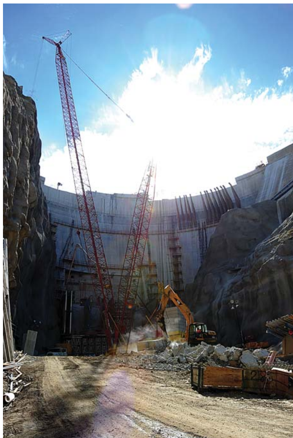
The Big Tujunga Dam is under construction to reinforce the walls due to an increased debris flow from recent severe winter storms, La Canada Flintridge, Calif., 2 August 2010. (Adam DuBrowa, FEMA)
