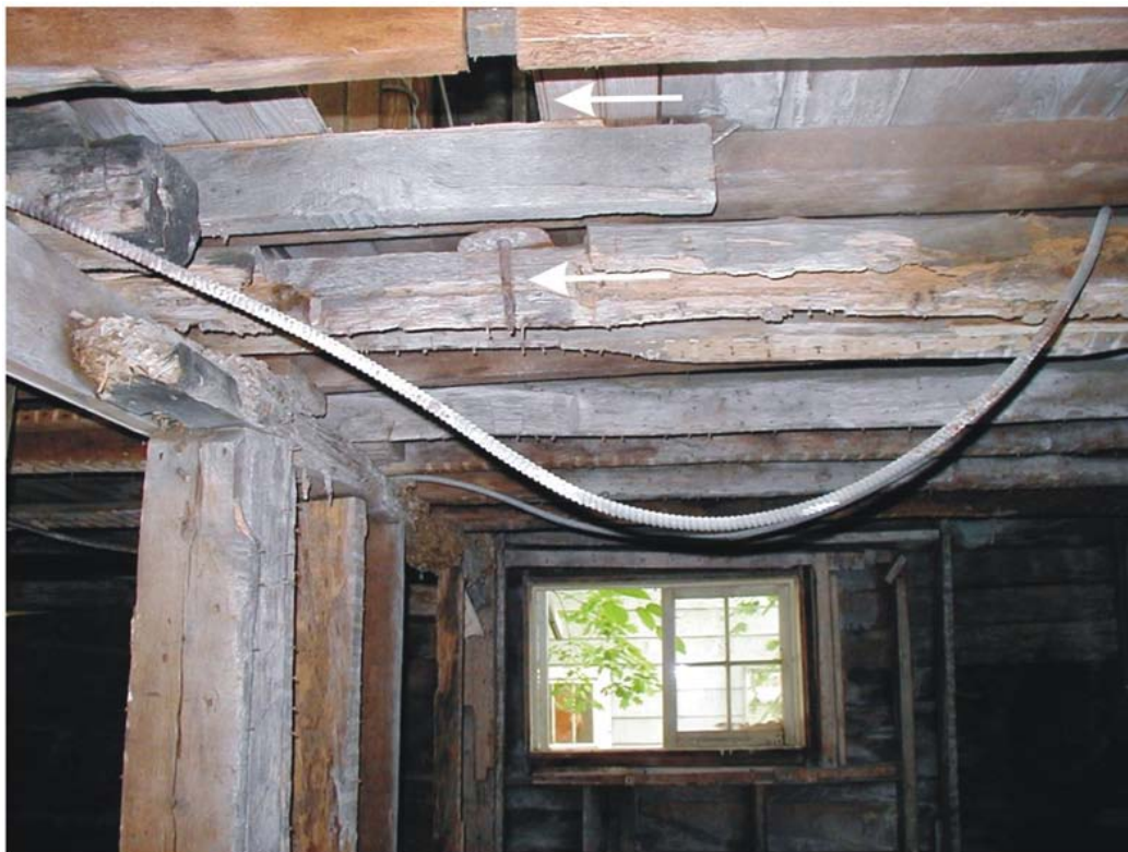
Figure 4. Hoe blade in situ. The upper arrow points to the hole in the second floor for the no longer extant chimney; the lower arrow points to the hoe blade, June 12, 2009 (Photo by Megan E. Springate).
