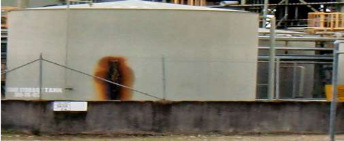
Fig 12: Cyanide leakage at the mining site
