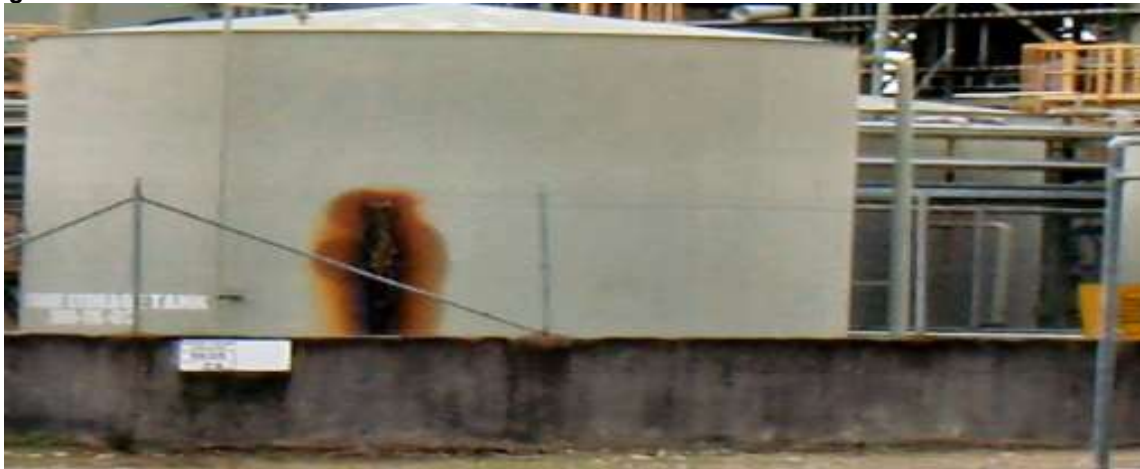
Fig 12: Cyanide leakage at the mining site
