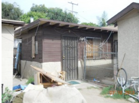
Rear patio converted into an unpermitted dwelling unit in unincorporated South Central Los Angeles
