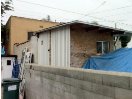
Unpermitted garage conversion with added living space in unincorporated South Central Los Angeles
