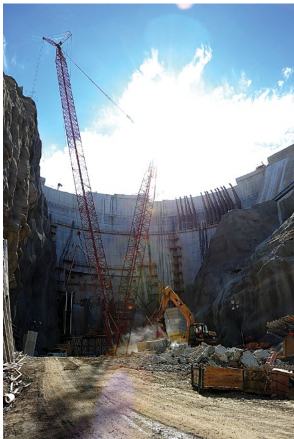
The Big Tujunga Dam is under construction to reinforce the walls due to an increased debris flow from recent severe winter storms, La Cañada Flintridge, Calif., 2 August 2010. (Adam DuBrowa, FEMA)
